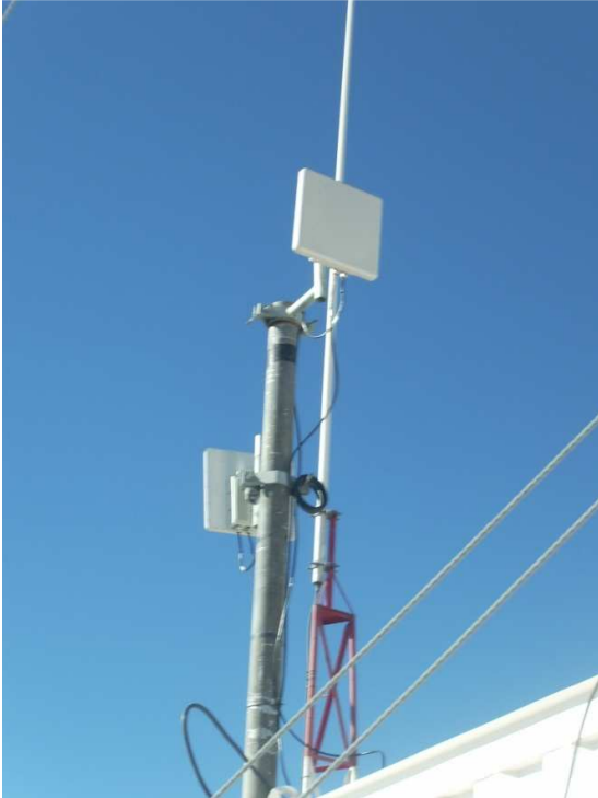
RADWIN 2000 high-capacity link deployment
