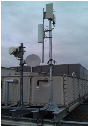
RADWIN 5000 deployment by BBnet, ISP in Ireland
